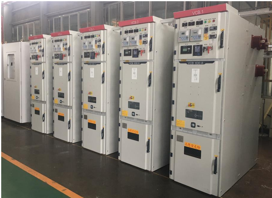
New Taipei city project -New substation
